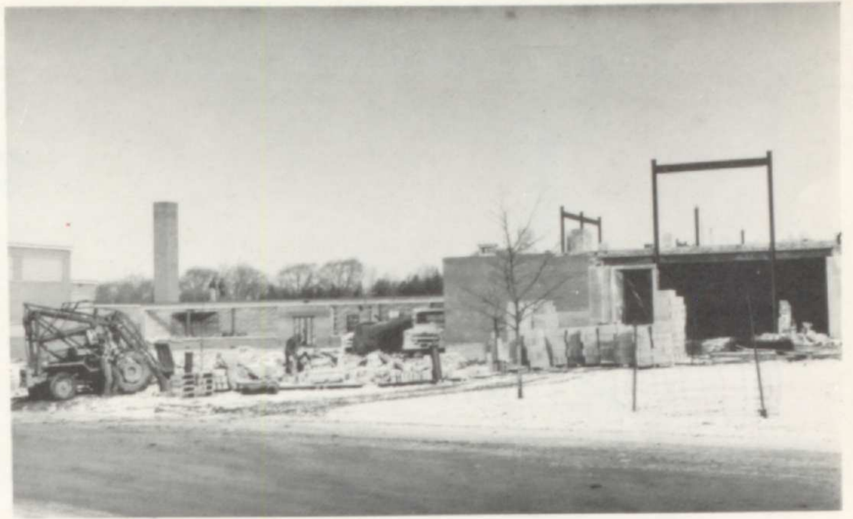
CONSTRUCTION —A picture of the new junior high school being added to the present building. At the other end of the school a music section is under construction.
