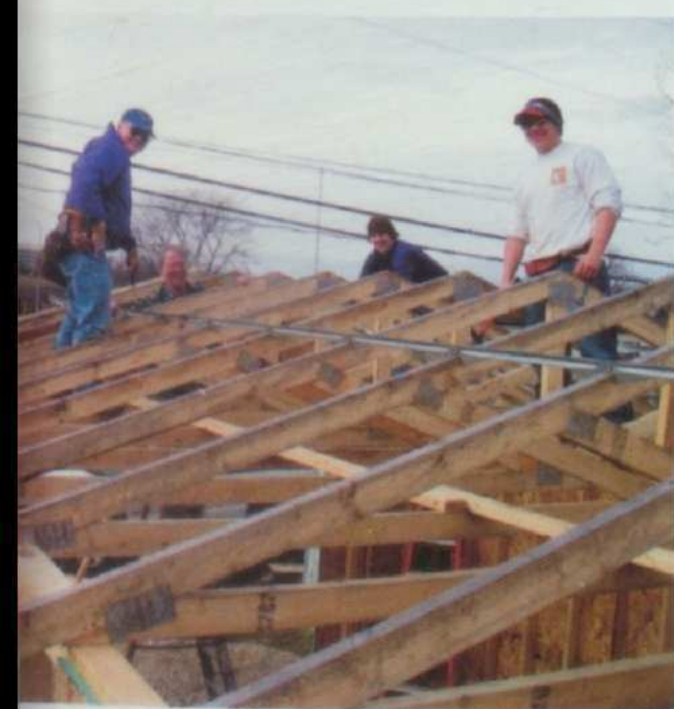
Above: Ben Willis and Andy Wolford are working along side mentors on preparing the roof of the garage for shingling.
