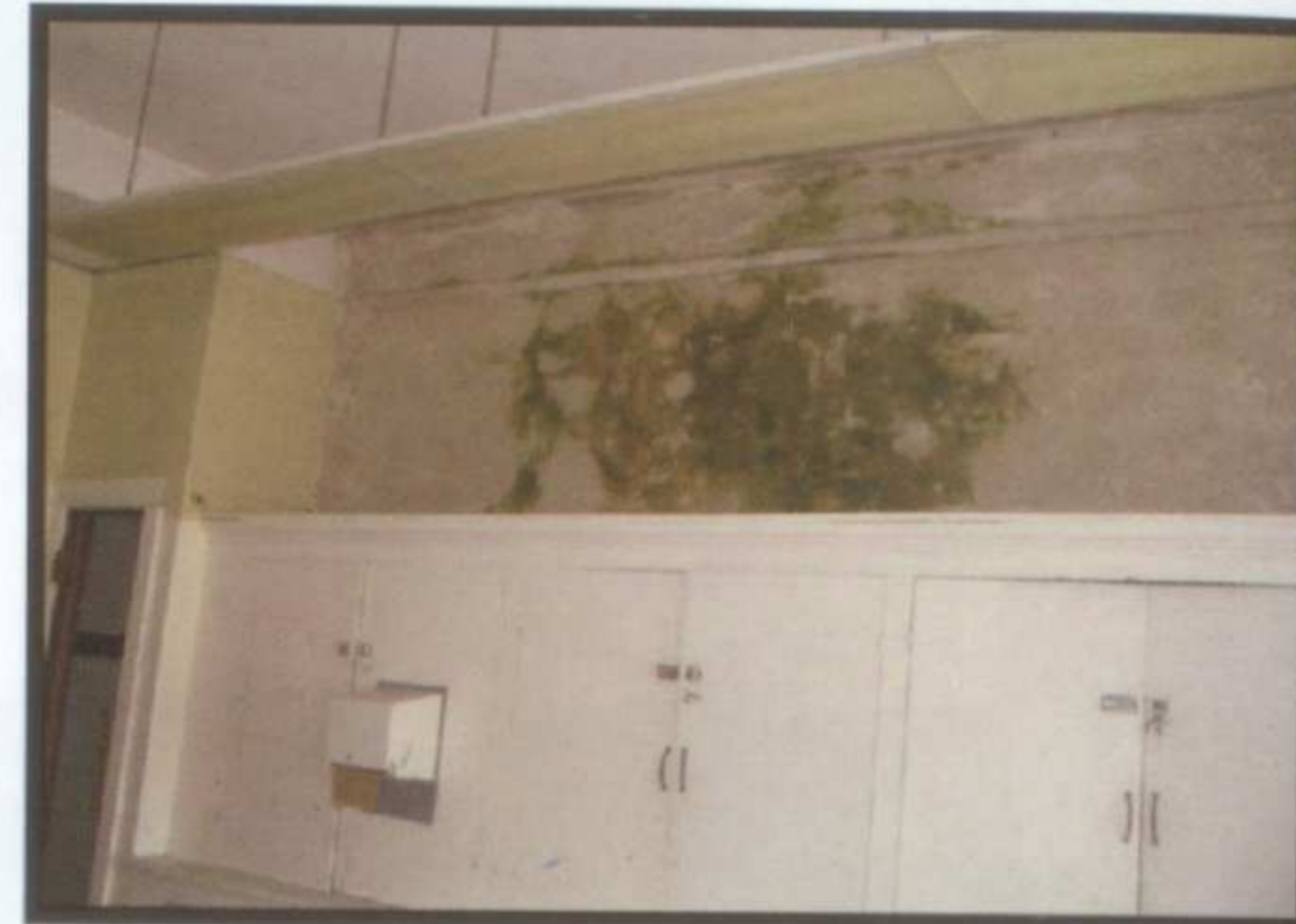
The walls of the Annex are covered in green mold from being damp throughout the years.
